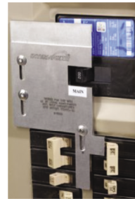
Generator Interlock Switch
